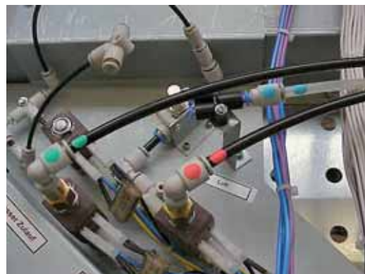
Abb. 8-8 Pipes at the nozzles
